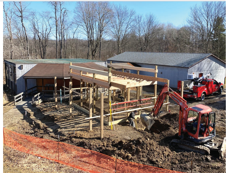
This photo shows the project progress as of mid-March. Construction has been happening quickly.
